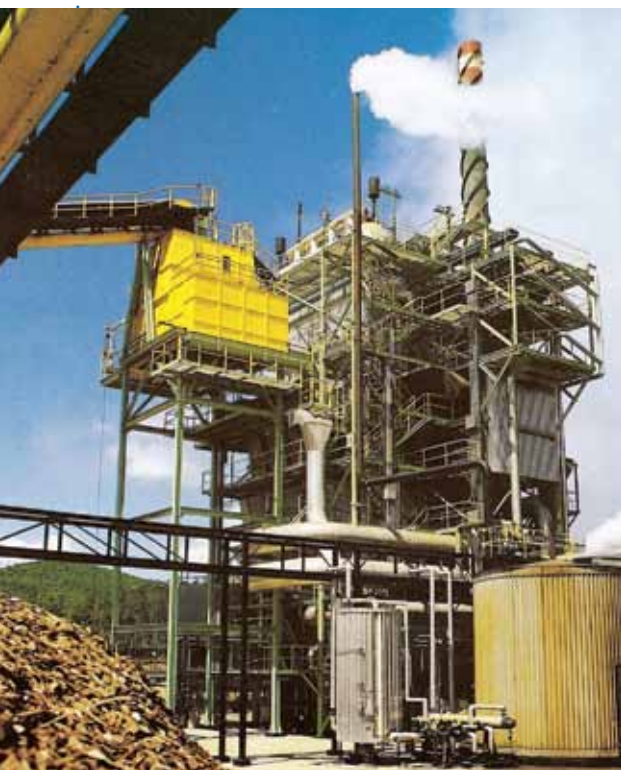
▼ Boiler burning wood chips
